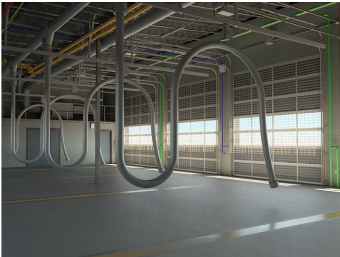
Left: Diesel Exhaust system a modern health and safety requirement.
