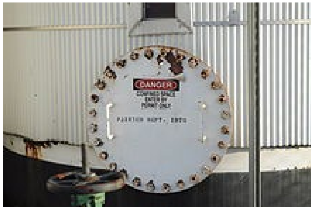
Left: A warning label on a storage tank, indicating that it is a confined space.
